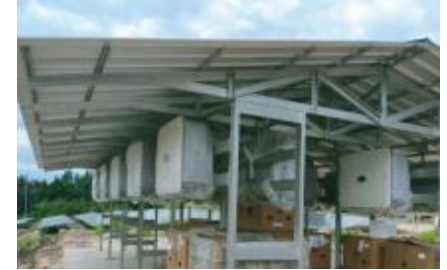
Inverters control panel
